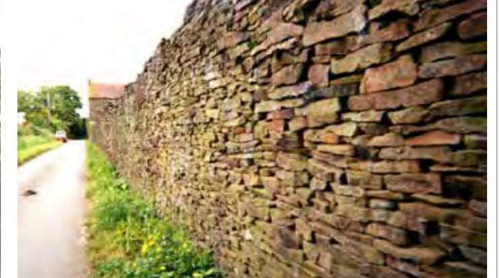
7 Looking north east along Mission Road. An example of a high, long, dry stone wall.
